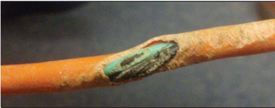
Figure 2: An electrocution incident and layout of the breeding and gestation barn where the incident occurred are described in Figure 1. The damaged area of the 100-foot extension cord is shown. This type of damage suggested that rodents had chewed the cord's outer insulation, allowing the flow of current through the metal of the pens and stalls.
